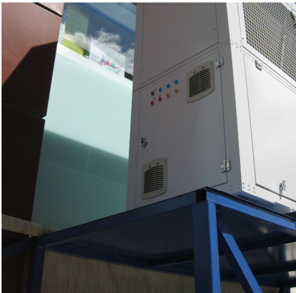
Missing rain or moisture protection at air entry to an outdoor electrical enclosure.
