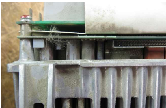
Dirt in enclosure contaminating FrigoPack
