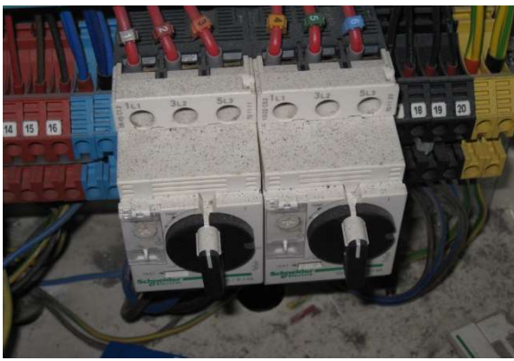
Dirt on all switchgear, Open hole in base
