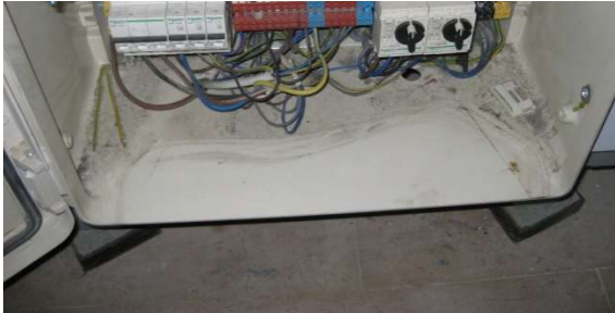
Unacceptable dirt build-up in enclosure
