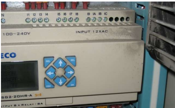
Fan blowing in wrong direction, dirt build up.
